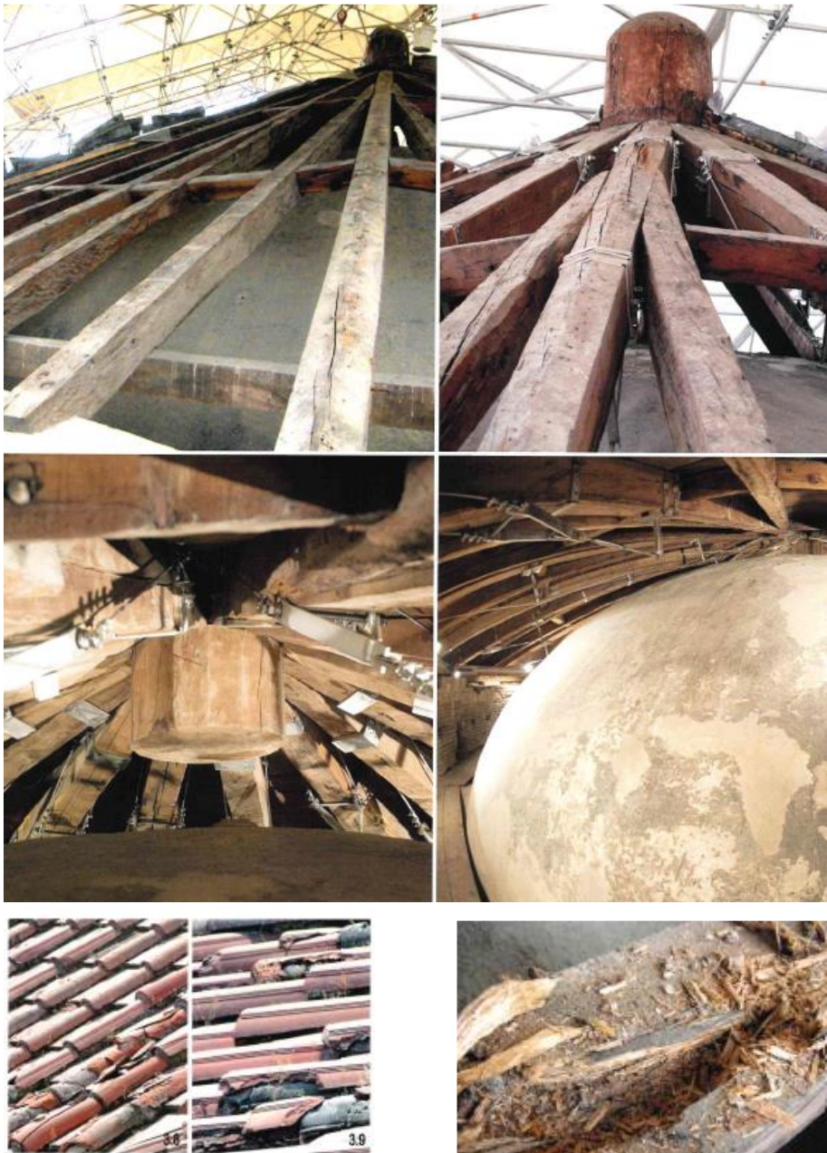
Restoration of the roof over the dome by arch. P. Focaccia. The state of structures and materials before and after the restoration. P. Focaccia, San Vitale , op. cit in references.
