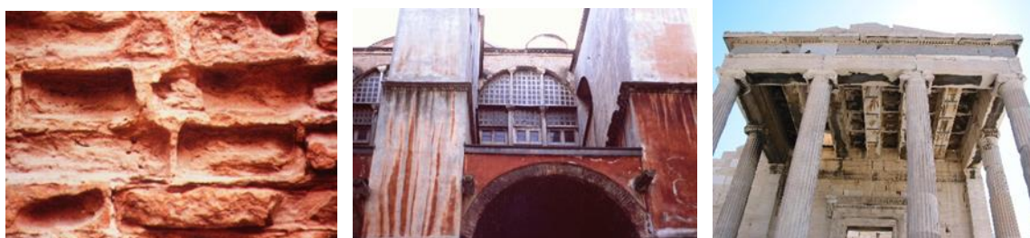
From left to right: Erosion; Decoloration; Black crust. Pictures by Nora Lombardini
